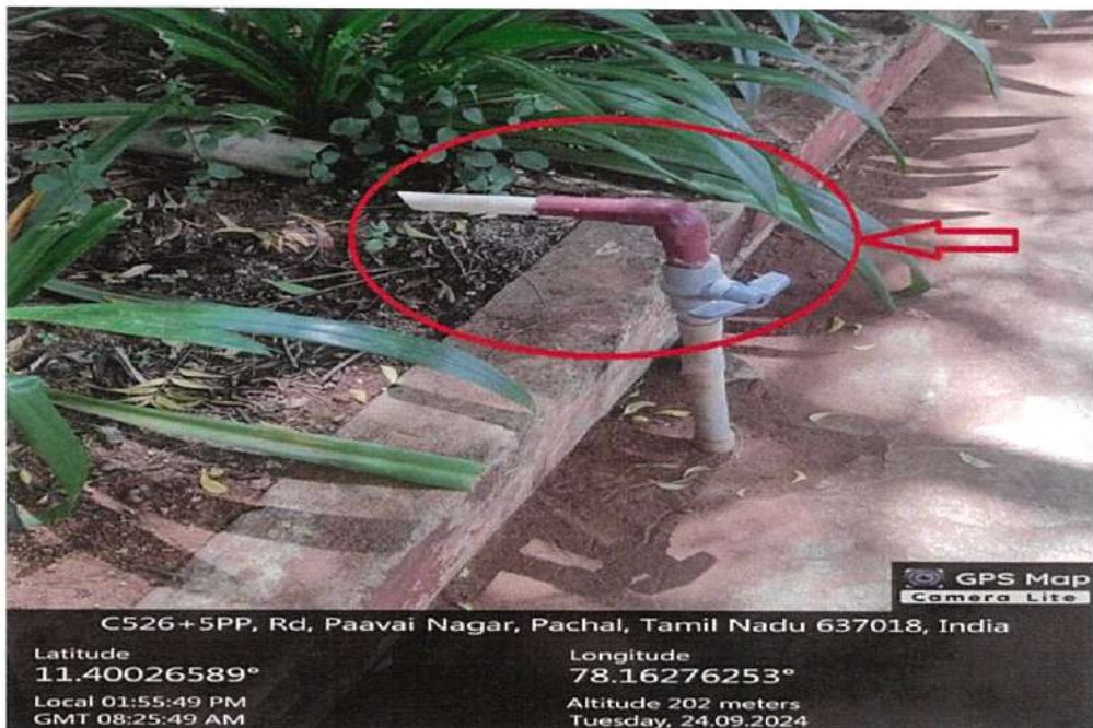
Reclaimed Water Supply Pipeline 2 in front of Main Block
