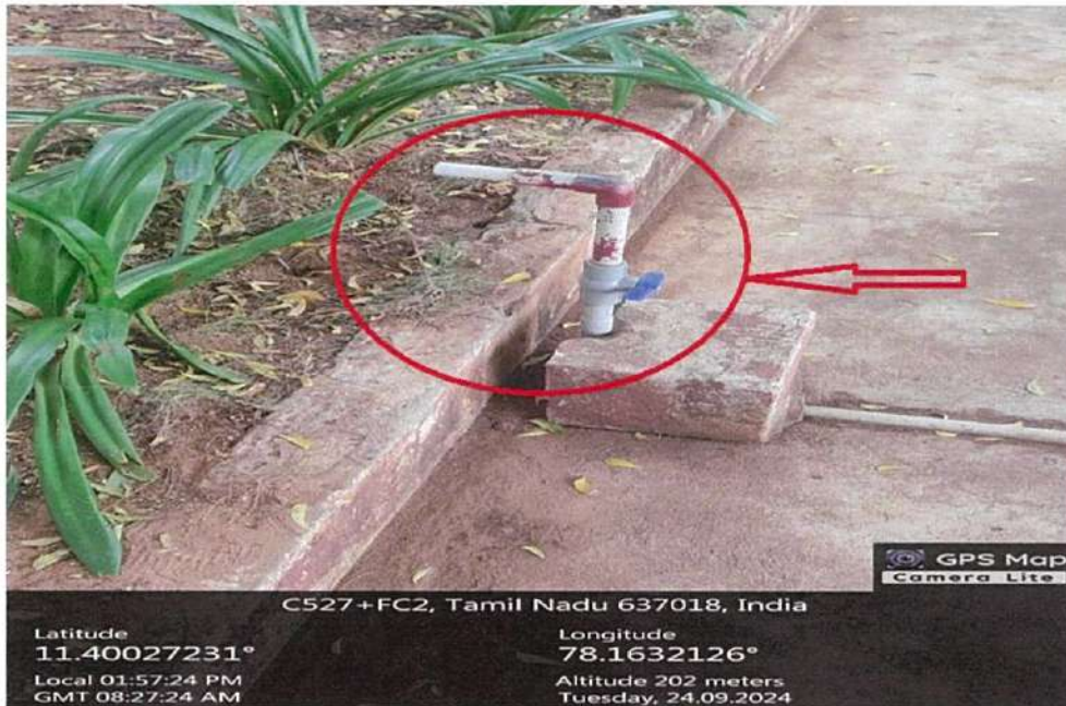
Reclaimed Water Supply Pipeline 3 infront of Main Block
