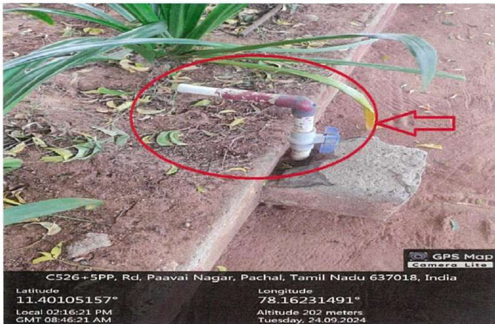
Reclaimed Water Supply Pipeline 2 in front of Arjun Maidan
