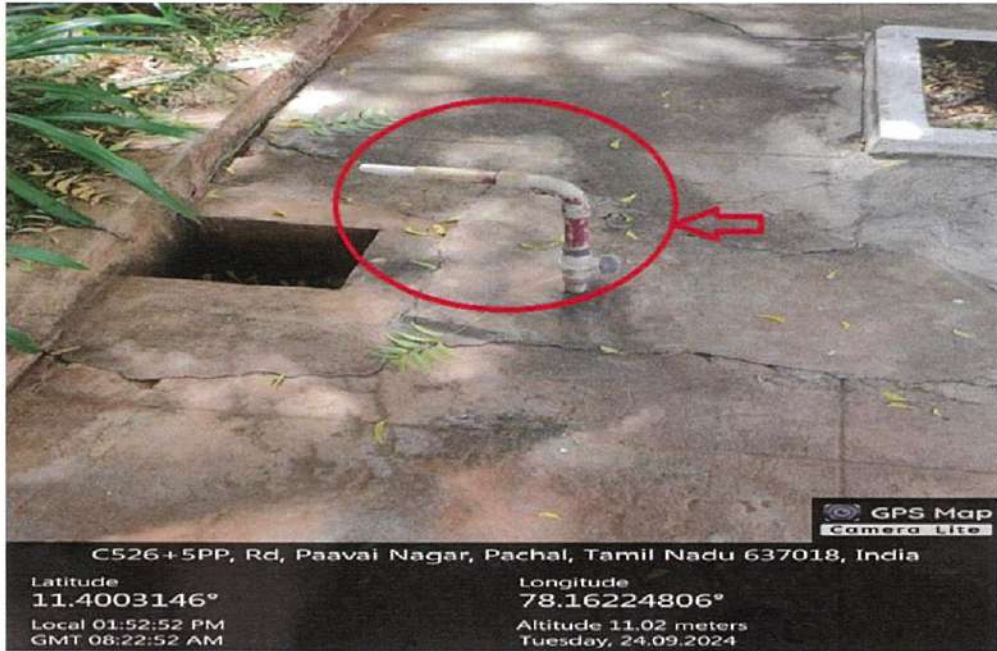
Reclaimed Water Supply Pipeline 1 in front of Arjun Maidan
