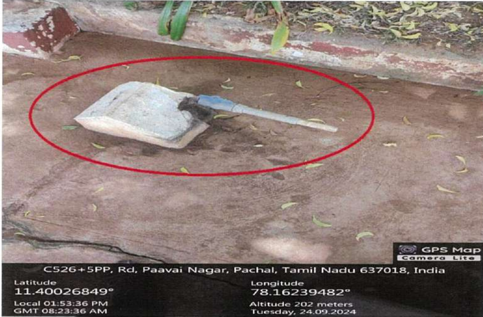
Reclaimed Water Supply Pipeline 1 in front of Main Block
