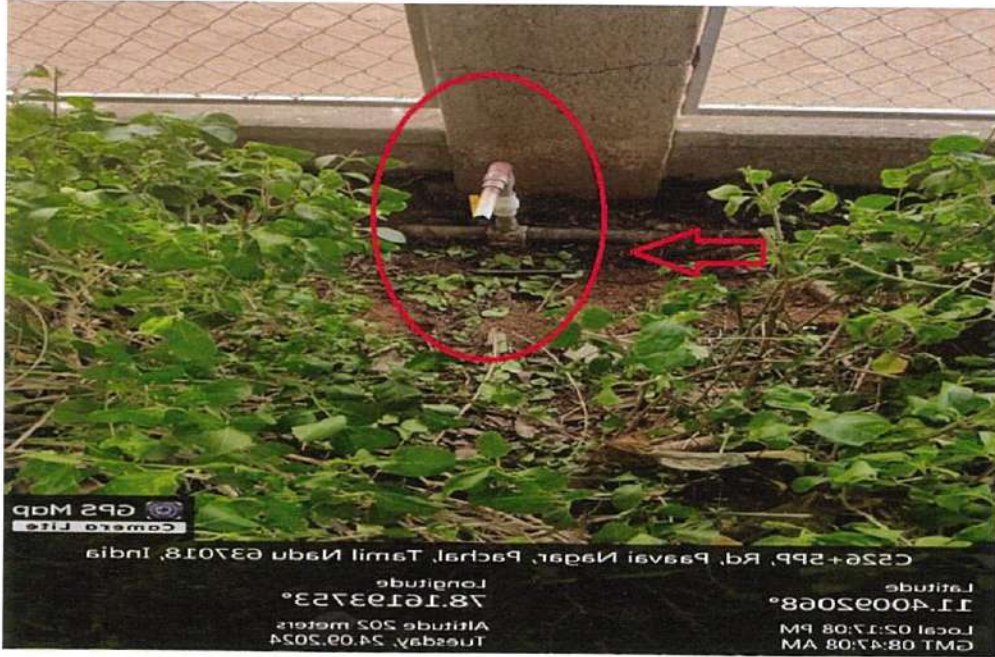
Reclaimed Water Supply Pipeline 1 opposite Arjun Maidan
