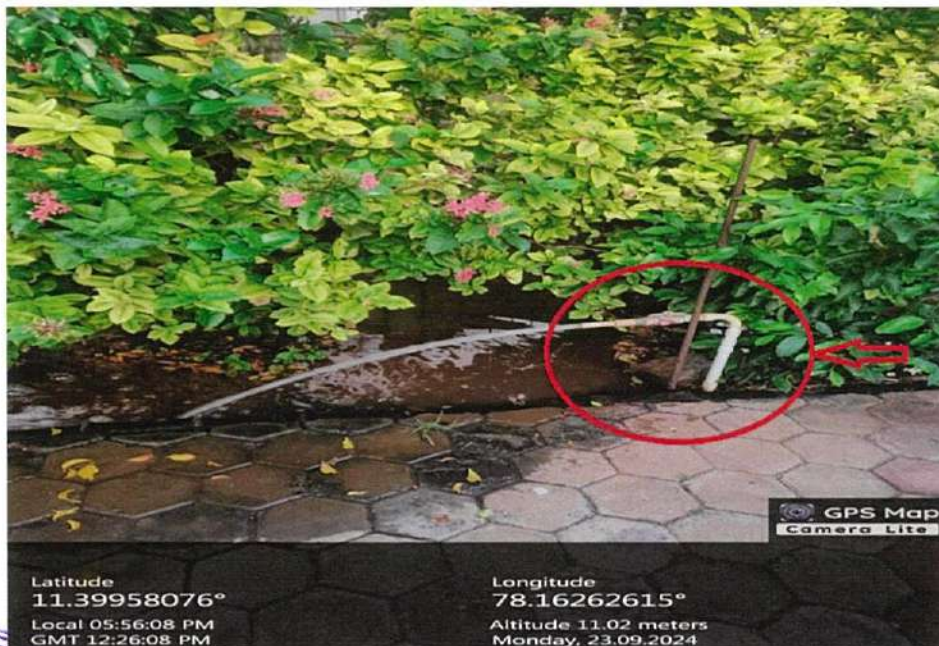
Recycled Water Supply to the plant
