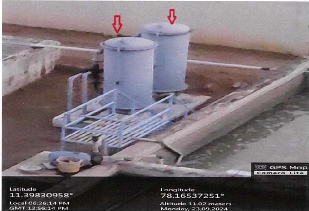
Sand Filter with Activated Carbon
